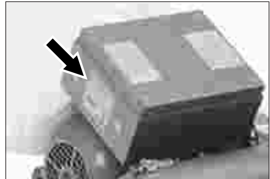
Fig. 3 Motor type plate on switch box.
